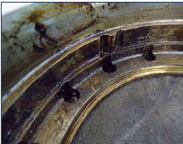
Dry Gas Seal contamination caused by ingress of unconditioned seal gas
