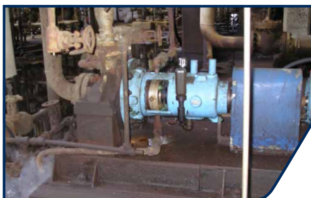
Legacy API pump with single seal installed
