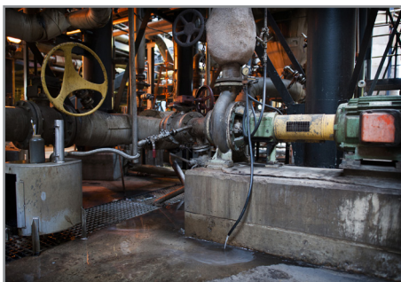
Before: Pump and mechanical seal at Mondi Richards Bay, fitted with quench-to-drain flushing system.
