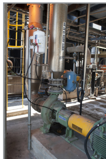
After: Pump and mechanical seal at Mondi Richards Bay, fitted with AESSEAL® continuous loop flushing and lubricating system.
