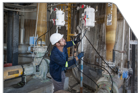
Continuous loop flushing and lubricating systems supplied by AESSEAL®, fitted to pumps at Mondi Richards Bay.
