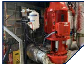
after - no leakage
