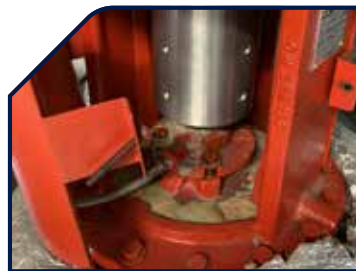
before - contamination leakage
