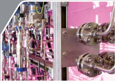
Dry gas seal support system
